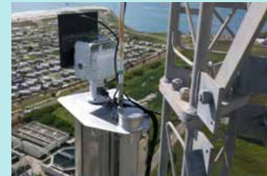
Communication Tower to transmit the remote control commands.
